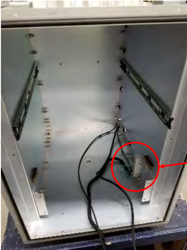
VR125 IP66 rated Cabinet (VR125 removed)
